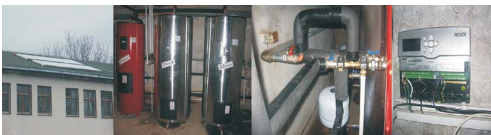
Figure 7. Details of installed equipment on the hospital from left to right: TS collectors; one tank of 500 l and two tanks of 1000 l; 3-way valve; monitoring system
