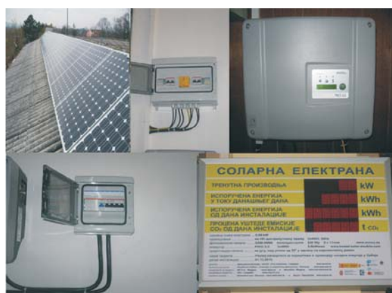
Figure 5. Details of installed equipment on the schools from left to right: PV modules; DC switching panel; Inverter; AC switching panel; Monitoring board (full color figure is available in electronic version)
